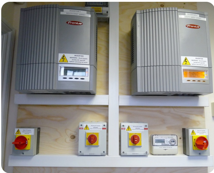
The dual inverters, switchgear and generation meter
