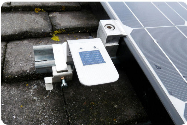
This small sensor, located next to one of the PV panels, records solar radiation intensity in W/m 2
