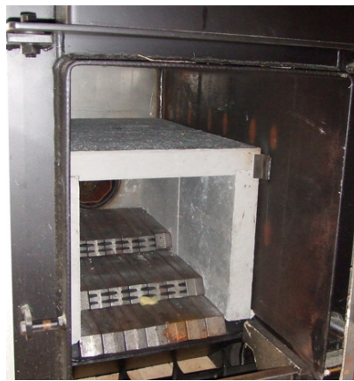
Moving grate in the fire box
