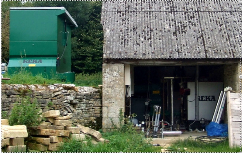
The 60kW Danish boiler installation, with hopper fuel store
