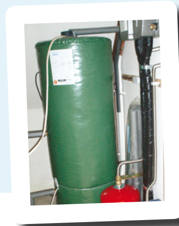
Well insulated cylinder connected to solar thermal and boiler
