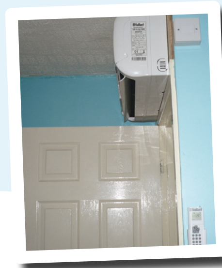
The air source heat pump system is operated with a remote control – seen in a wall mounted cradle.
