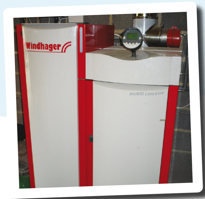
Wood pellet boiler and hopper
