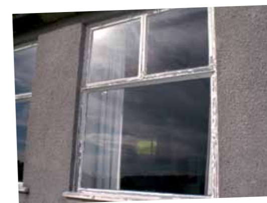
The pre-Target 2050 project single glazed metal frame windows contributing to heat loss
