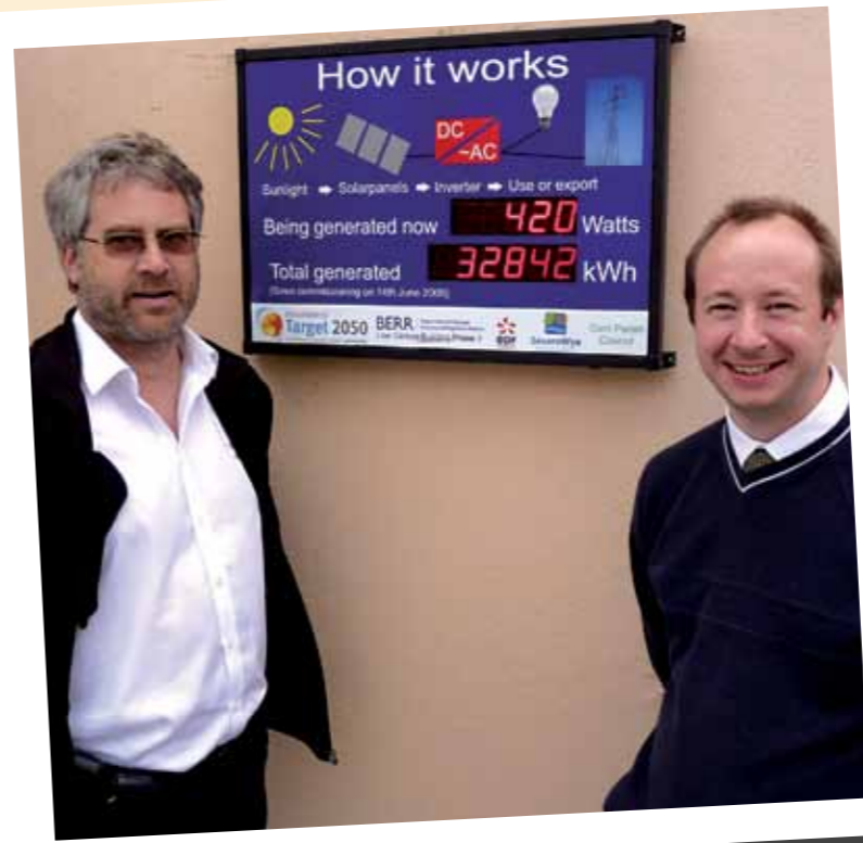
Members of the hall committee, Keith Pearce and Jeremy Clutterbuck, with the public facing display showing 'real time' performance of the solar photovoltaic system.
