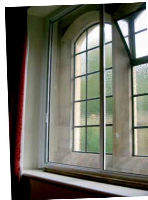
Secondary glazing installed in one of the participating halls – helping to keep heat in and cold draughts out
