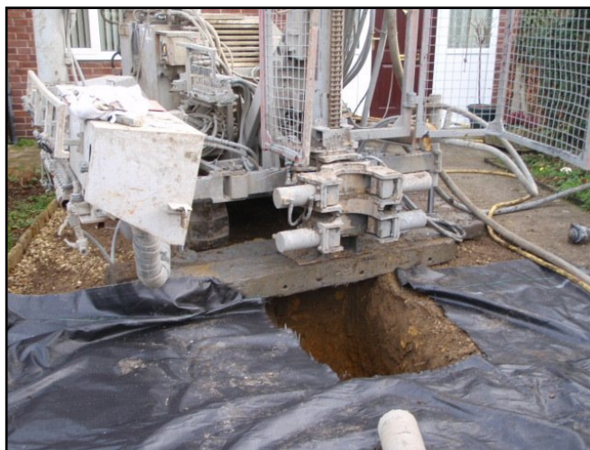
Sump pit to catch initial waste water (Picture courtesy of Stroud DC)
