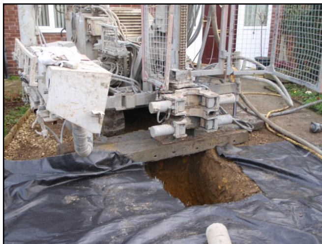
Sump pit to catch initial waste water (Picture courtesy of Stroud DC)
